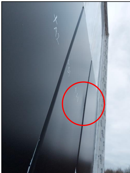
Photograph No. 3 – Damage caused following impact ref A1
