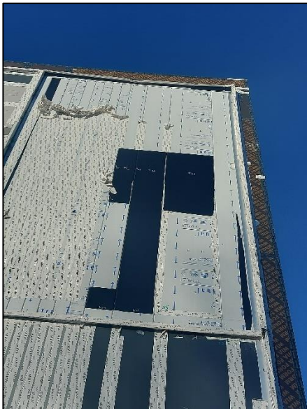
Photograph No. 15 - Top right hand corner panels
