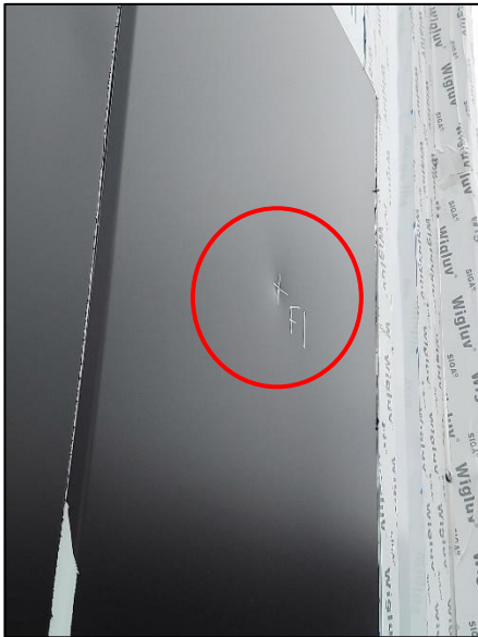
Photograph No. 8 – Damaged caused following impact ref F1
