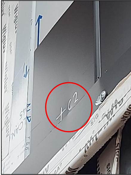
Photograph No. 7 – Damage caused following impact ref C2
